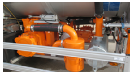
FIGURE 24: Ensemble pompe à vide + accessoires
